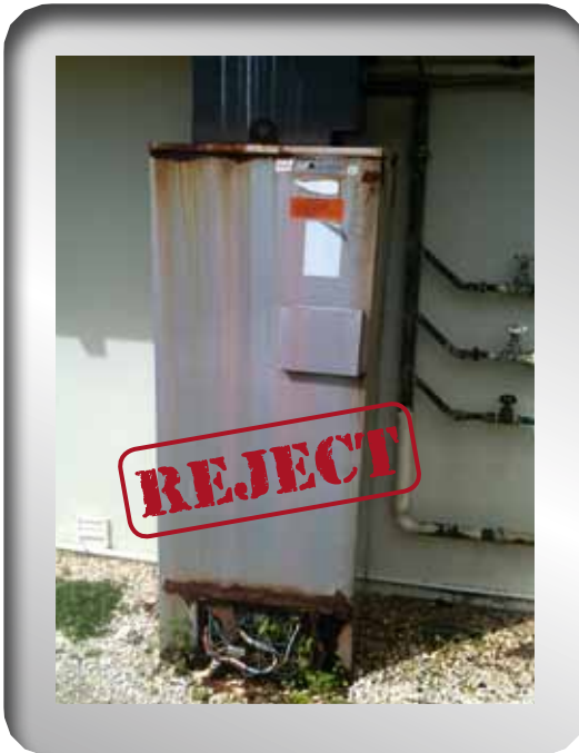
Corroded hot water units.
