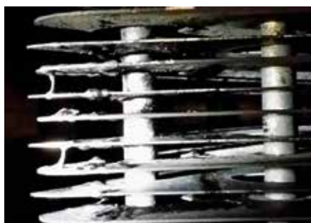
Figure 7: Extensive grease build-up on an ESP due to poor maintenance, directly connecting the charged and the ground plates and grounding the whole unit.
